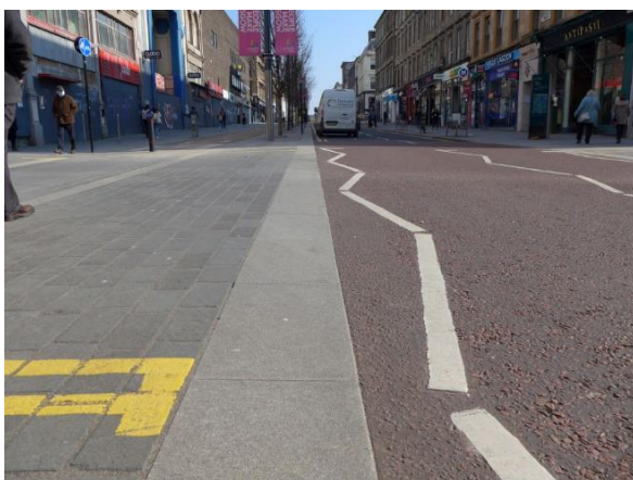
Lack of ramp at edge of main carriageway
